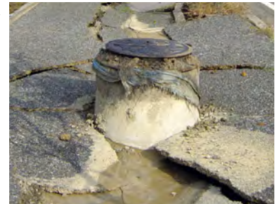
Manhole floats from liquefaction
