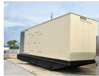
Power Supply and Electrical Components
